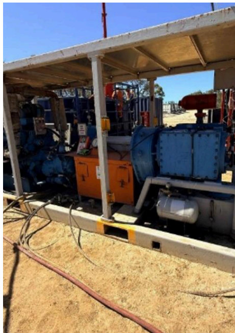
Skid pump with SPM triplex service pump
